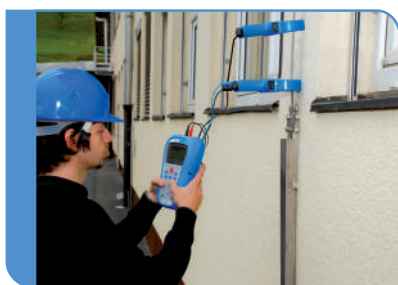
Two clamps method for testing ground resistance of object on TN system
